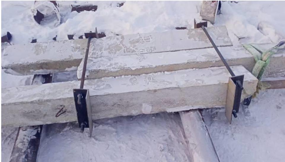
Fig. 5. The way of fastening the ballast to transfer the test load to the footings.
