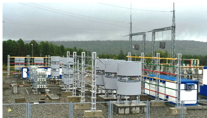
Fig. 6. A general view of two static var compensators at the Skovorodino OPS-21 of the Transneft-East LLC.
